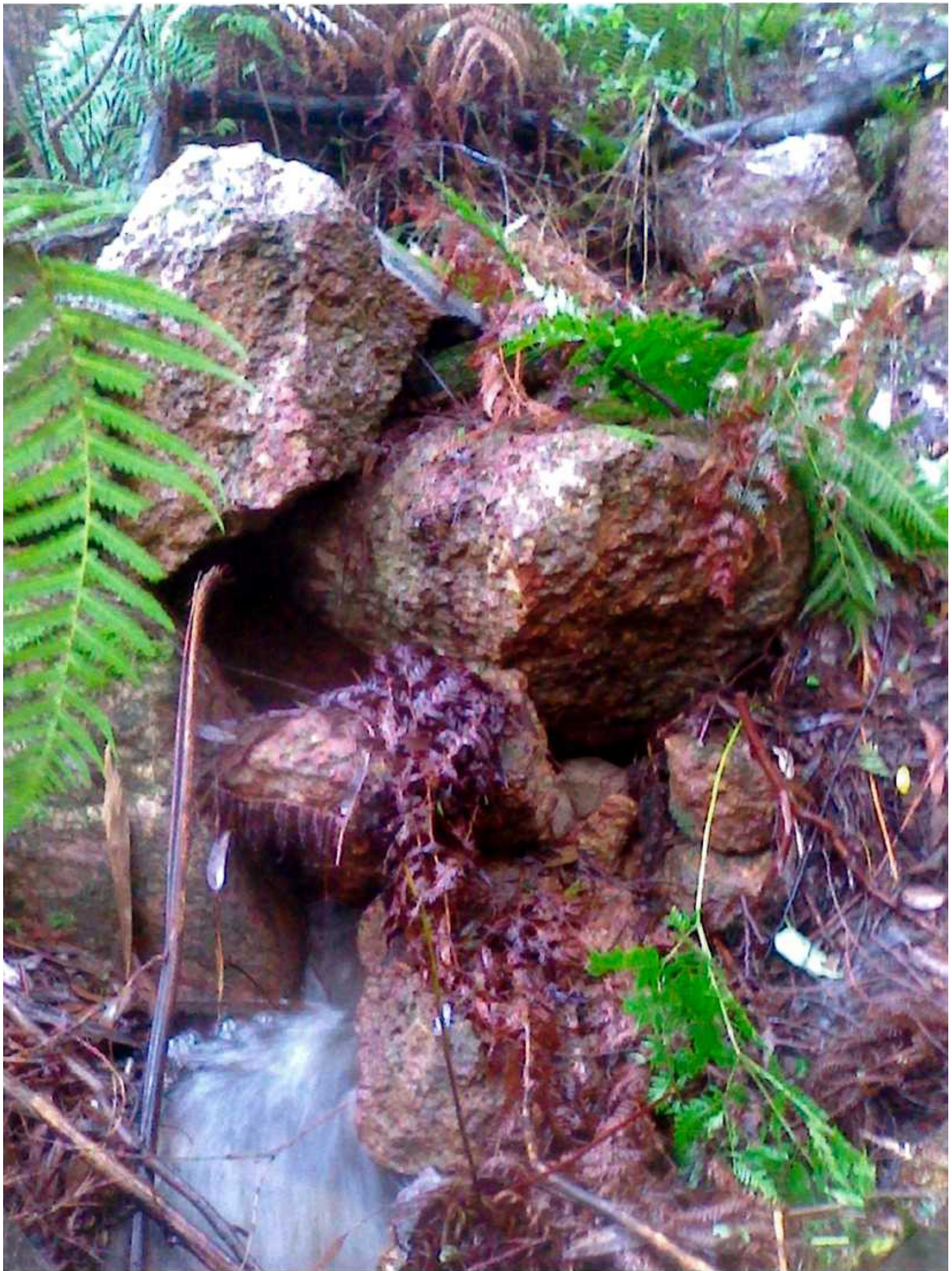
WATER RUNNING THROUGH THE EMBANKMENT SOUTH OF ROAD AND 100 FEET BELOW ROAD
