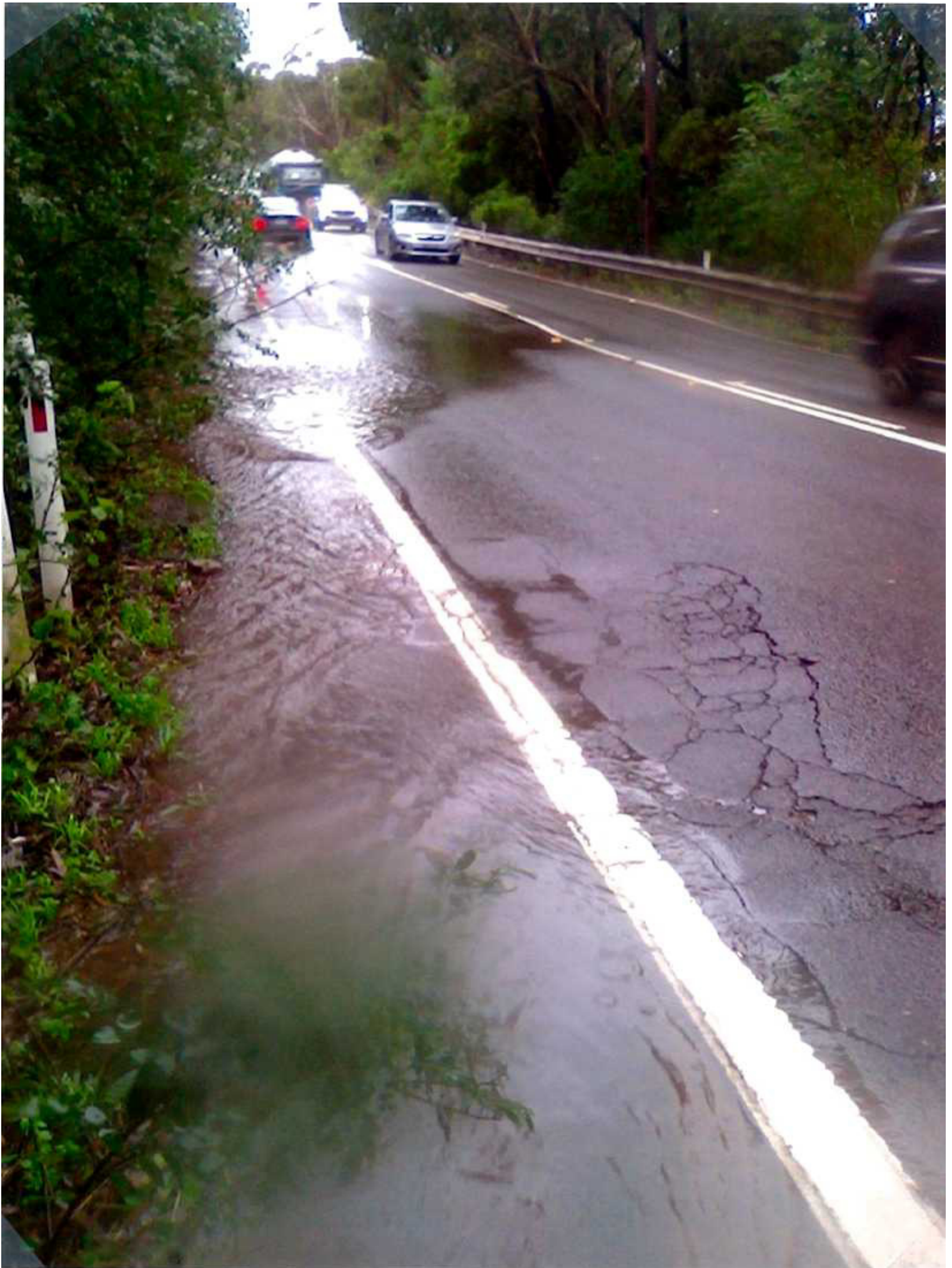
RUNOFF AND PUDDLE AT DIP EAST OF KIMBRIKI
