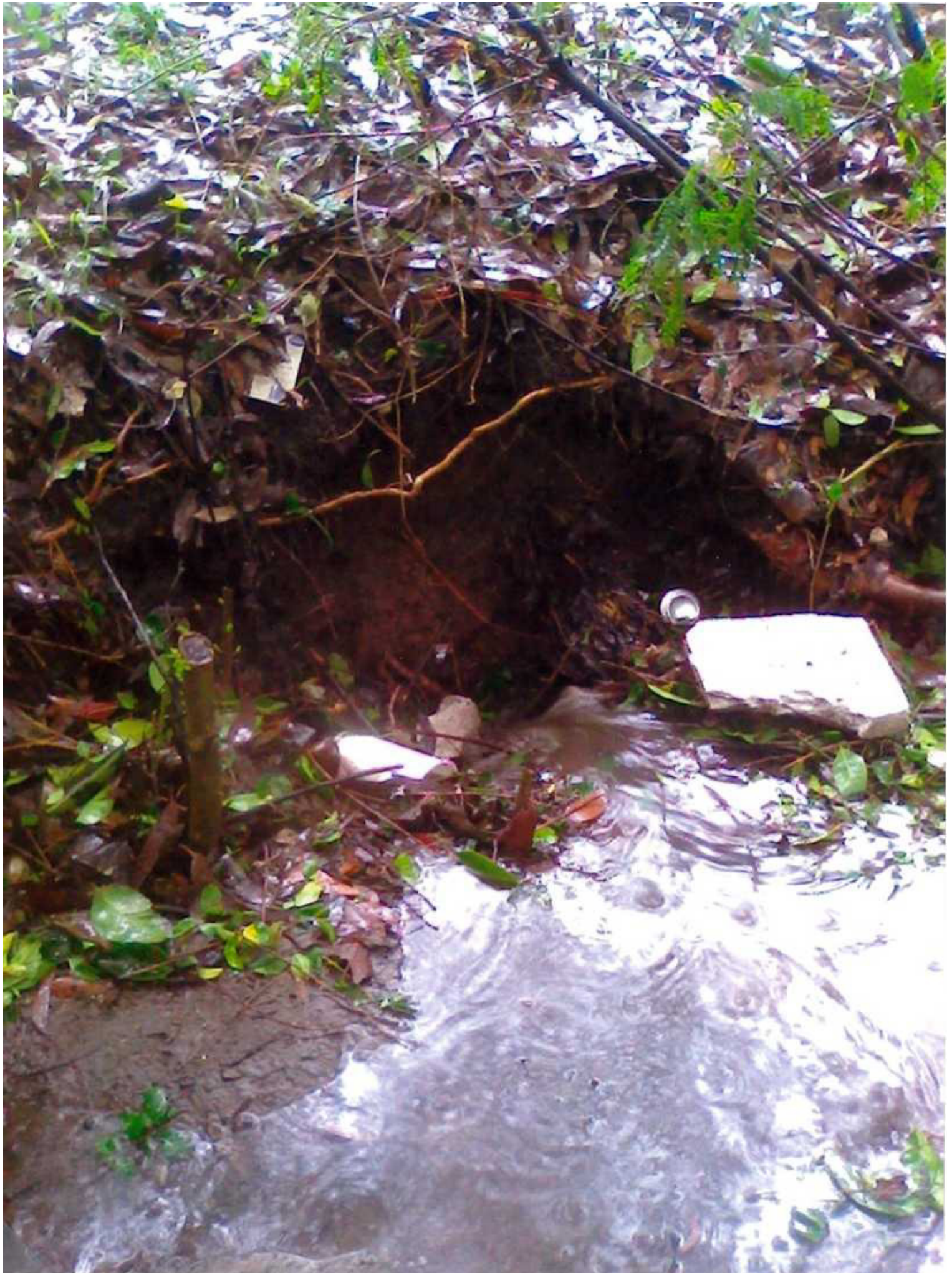
HOLE BESIDE ROAD 5 METRES EAST OF BLOCKED CULVERT WITH WATER RUNNING THROUGH THE ROAD EMBANKMENT 80 YEARS OLD
