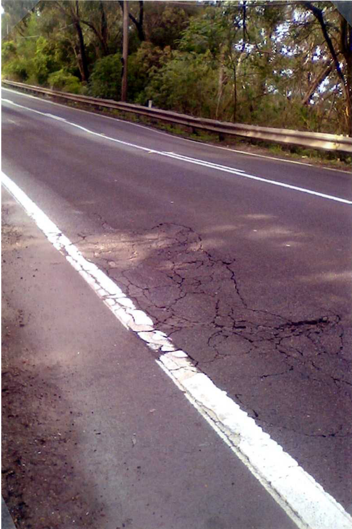
MONA VALE ROAD SUBSIDENCE 23.07.2022
